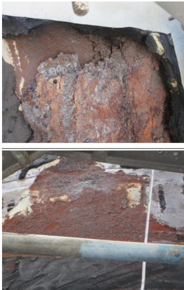
Figure 2. Corrosion state inspected on site
